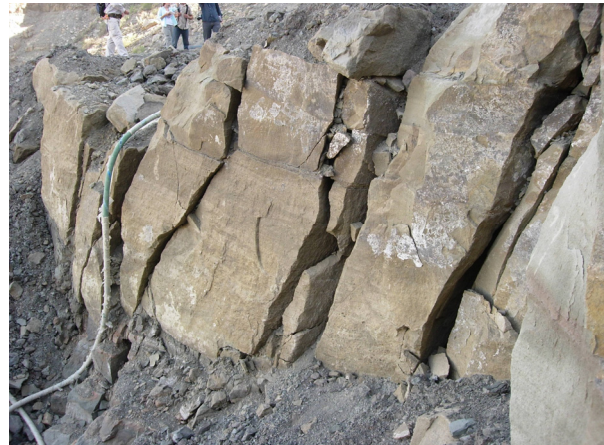
Figure 8b. Close up of figure 8a. Open joints are filled with pieces of rocks.
