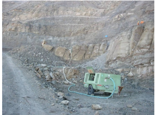
Figure 8a. Stepped and rotated block due to the slide process near portal of T3.
