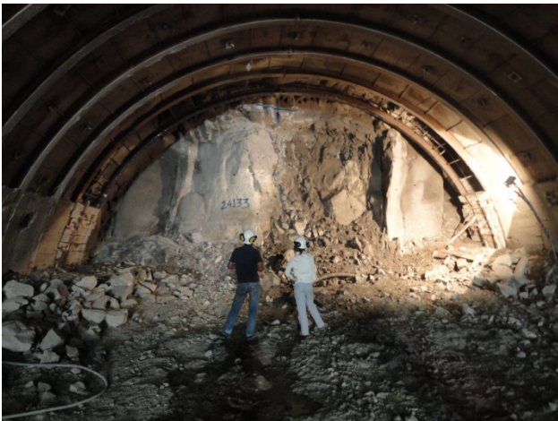
Figure 10. Cataclastic fill between rock blocks in T3.
