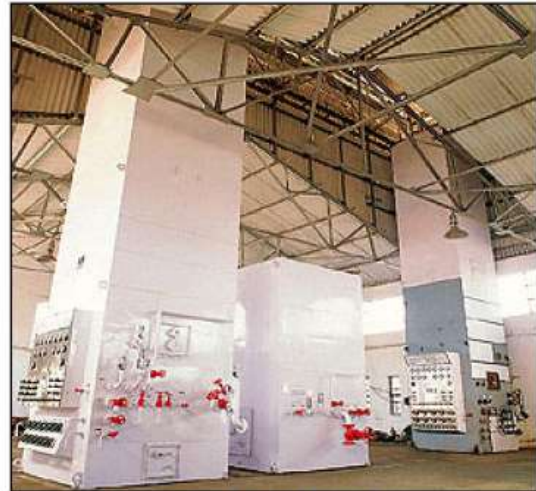
600 cu.m./hr. Oxygen Column
