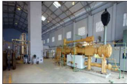
Air compressor for Oxygen Plant
