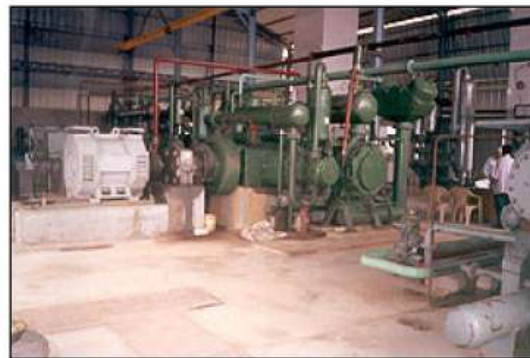
Nitrogen Compressor for 600 cum/hr Plant
